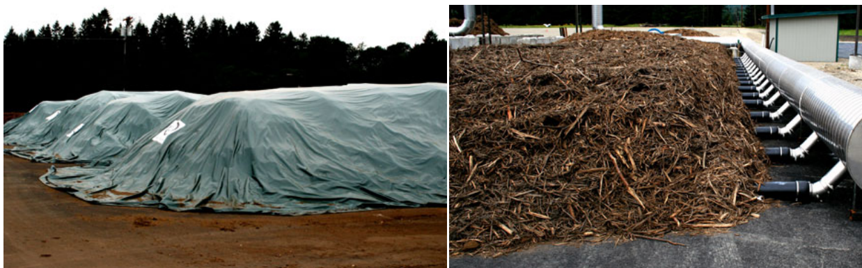
Figure II-1. Covered Negative-pressure ASP with Biofilter System
